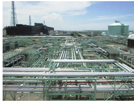
Photograph.1 C14 One part of facilities in Nihonkai LNG Niigata Terminal
