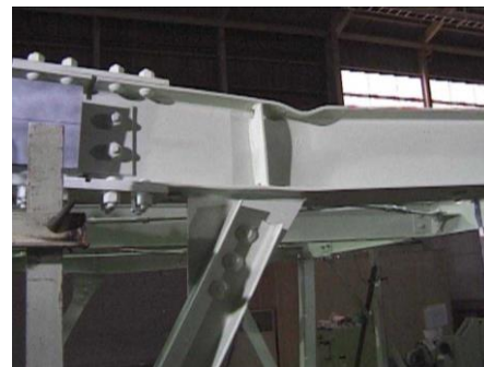
Photograph-6 The beams buckled by the static load experiment (Type-3)
